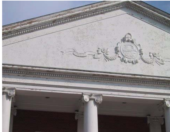
Problem- cracked, peeling paint on buildings. Short durability of existing coatings
